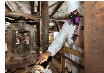
ASBESTOS CONTAINMENT AREAS
